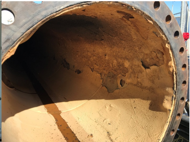
Above Ground Discharge Header
