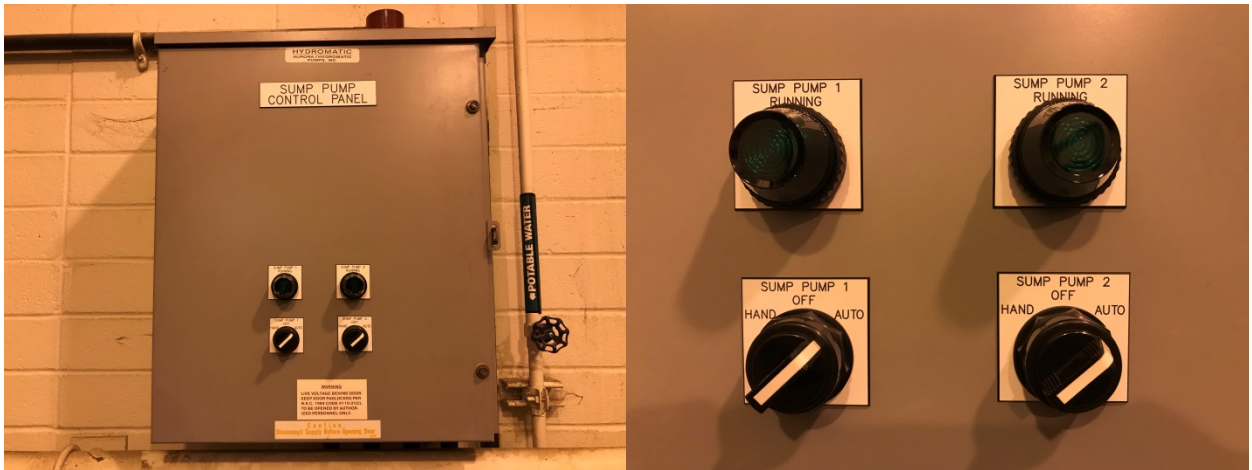
MDF SBS Building Sump Pump Control Panel – After Upgrade
