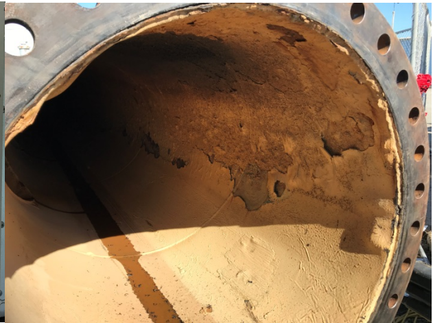
Above Ground Discharge Header
