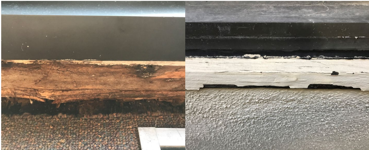
Dry Rot Inside The GM's Office
