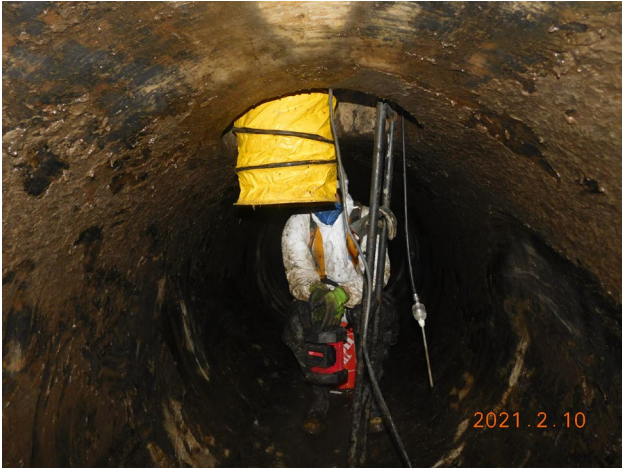
Inside Force Main
