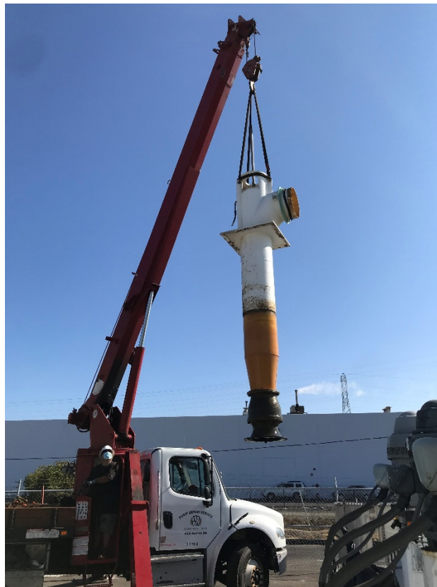
HEPS Effluent Pump No. 4
