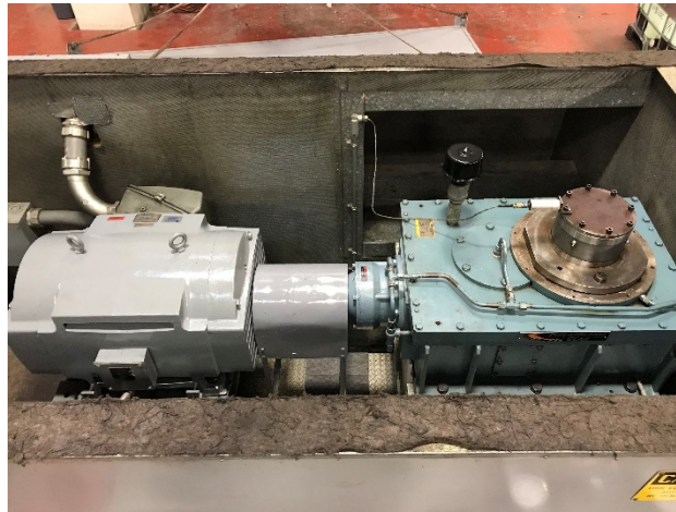
OLEPS Effluent Pump No. 4 Right Angle Gear Drive & Motor
