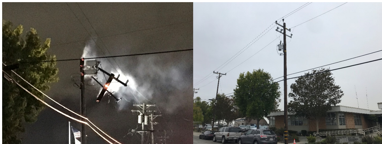
High Voltage Wires Supporting Pole Top
