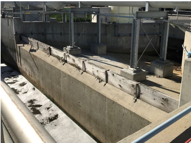
Old Lumber Emergency Outfall Weir
