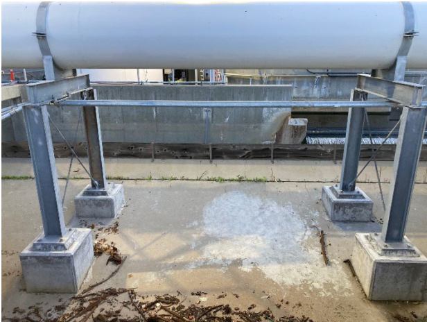
Old Lumber Weir & Expansion Joint
