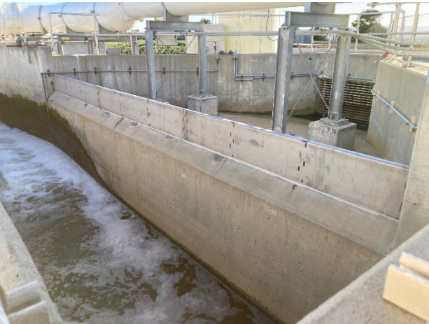
New Stainless-Steel Emergency Outfall Weir
