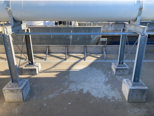
New Stainless-Steel Weir & Expansion Joint
