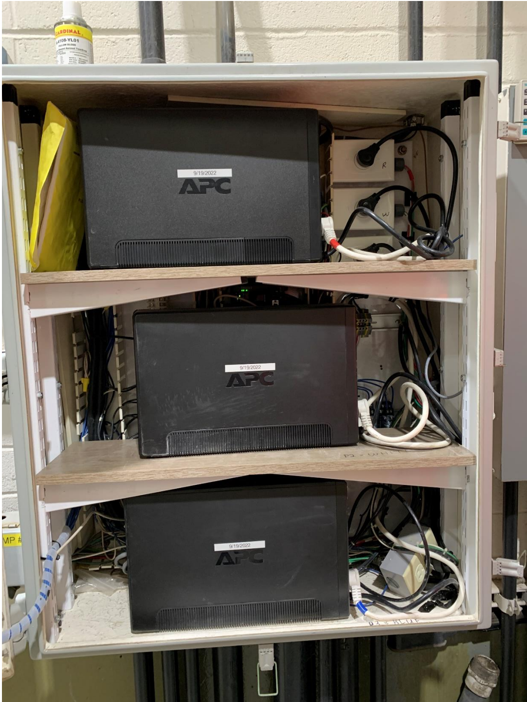
Figure 9. The three uninterruptible power supply boxes support the Facility’s programmable logic controller during a power outage. EBDA last replaced these in September 2022. According to the O&M Manager, the power supply boxes are replaced every four years.
