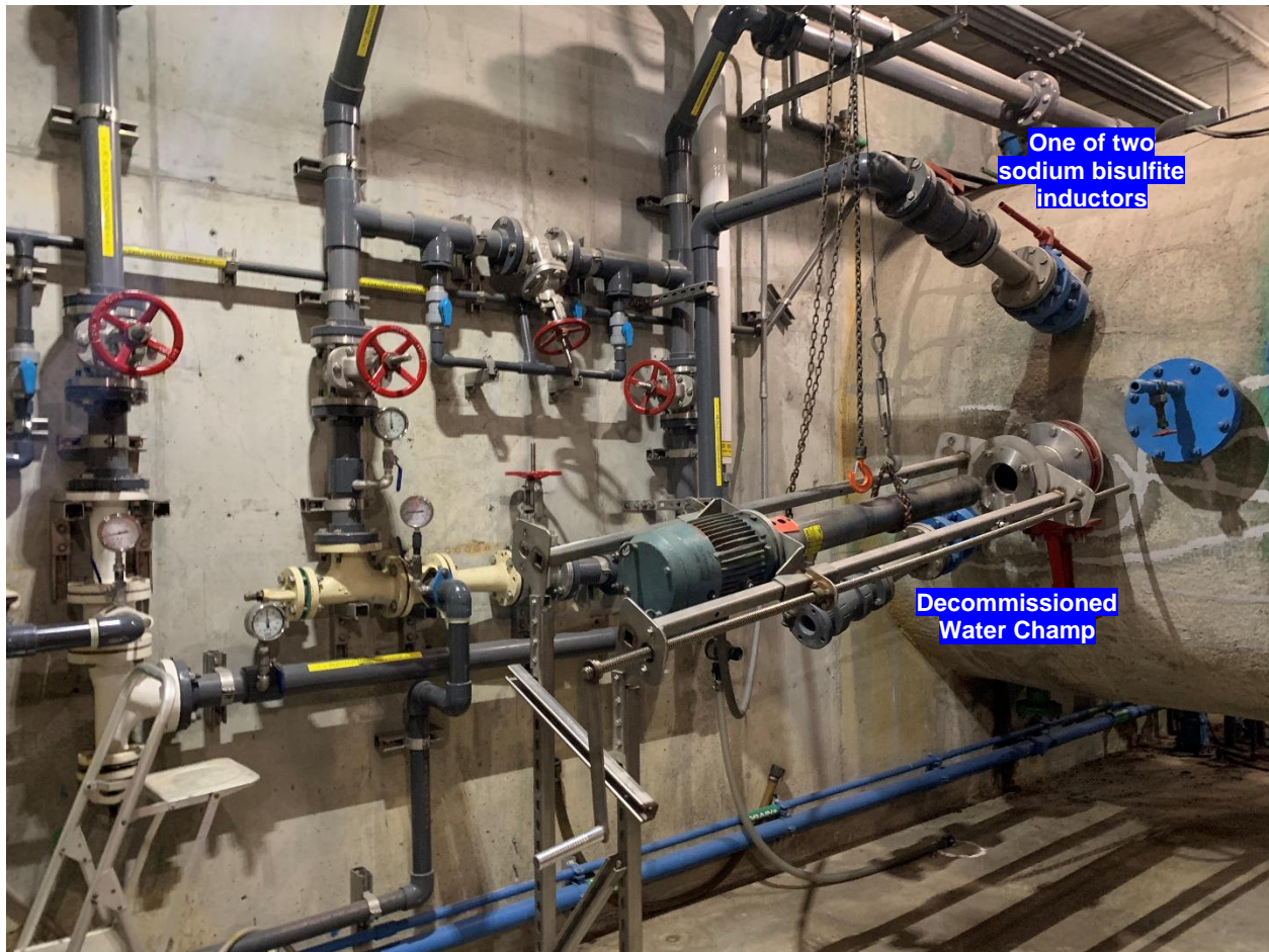
Figure 11. Sodium bisulfite is injected into effluent pipeline by two inductors immediately following the convergence of the two influent force mains. The decommissioned chemical mixer, or Water Champ, used to be EBDA's primary method of dechlorinating its effluent.
