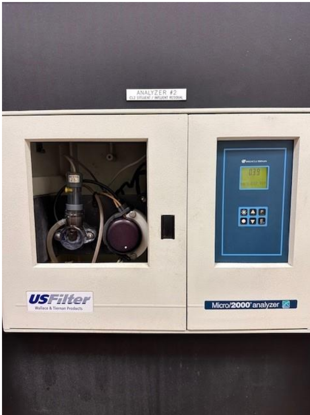
Figure 4. The effluent chlorine analyzer read 0.39 mg/L at the time of the inspection.
