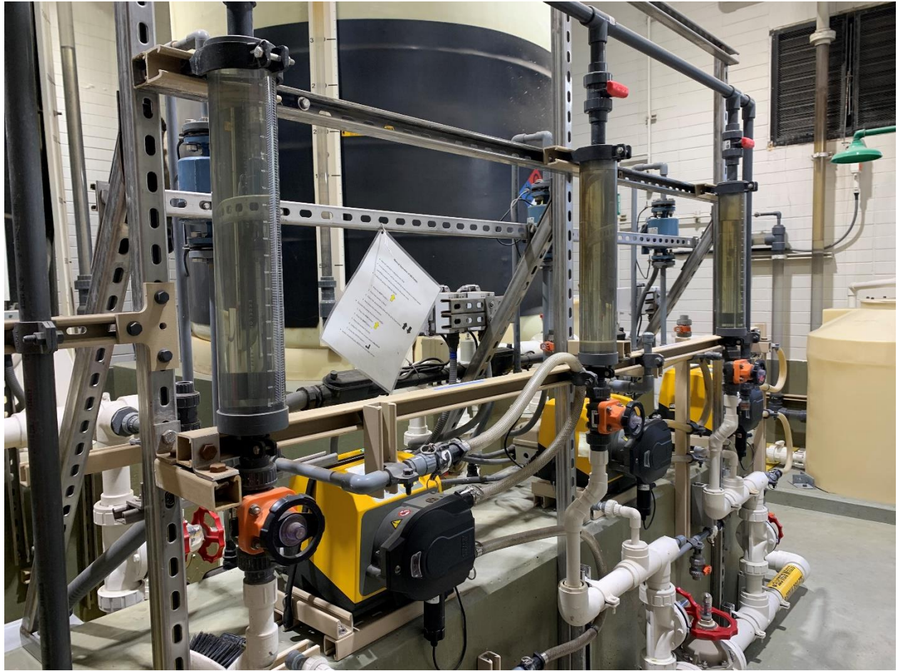
Figure 7. Three sodium bisulfite pumps.
