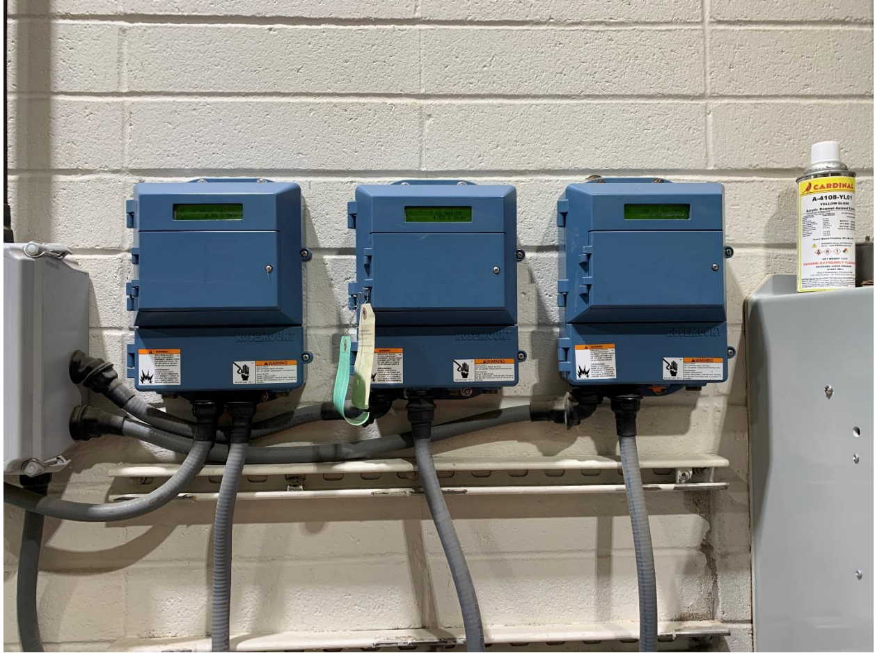
Figure 8. The three sodium bisulfite flow meters.
