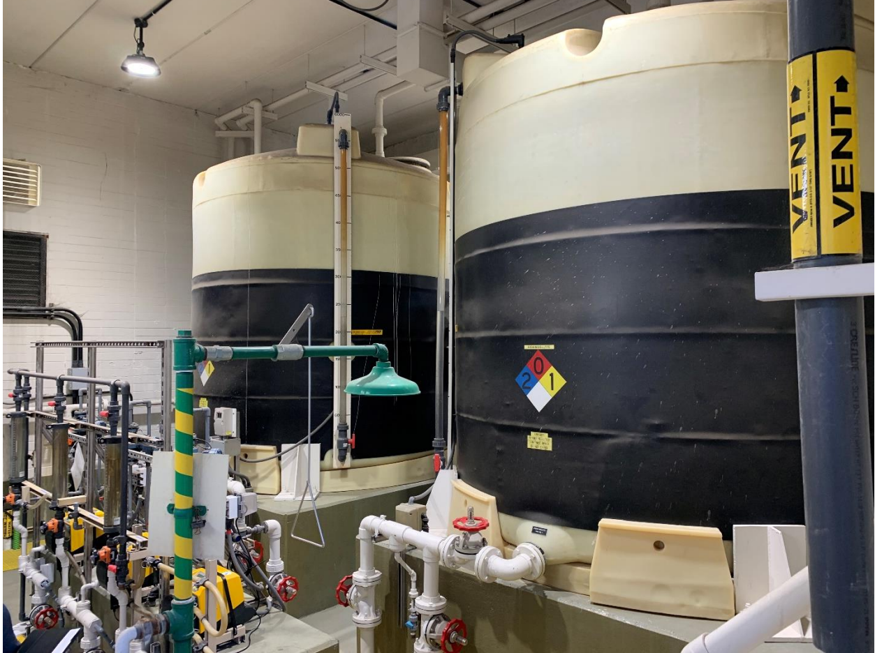
Figure 6. The Facility's sodium bisulfite storage building contained two 6,000-gallon tanks of sodium bisulfite.
