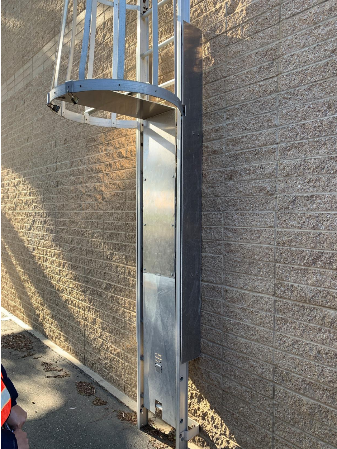
Figure 13. EBDA installed metal guards on the front and sides of the ladder to prevent people from climbing to the roof of the sodium bisulfite storage building after hours.
