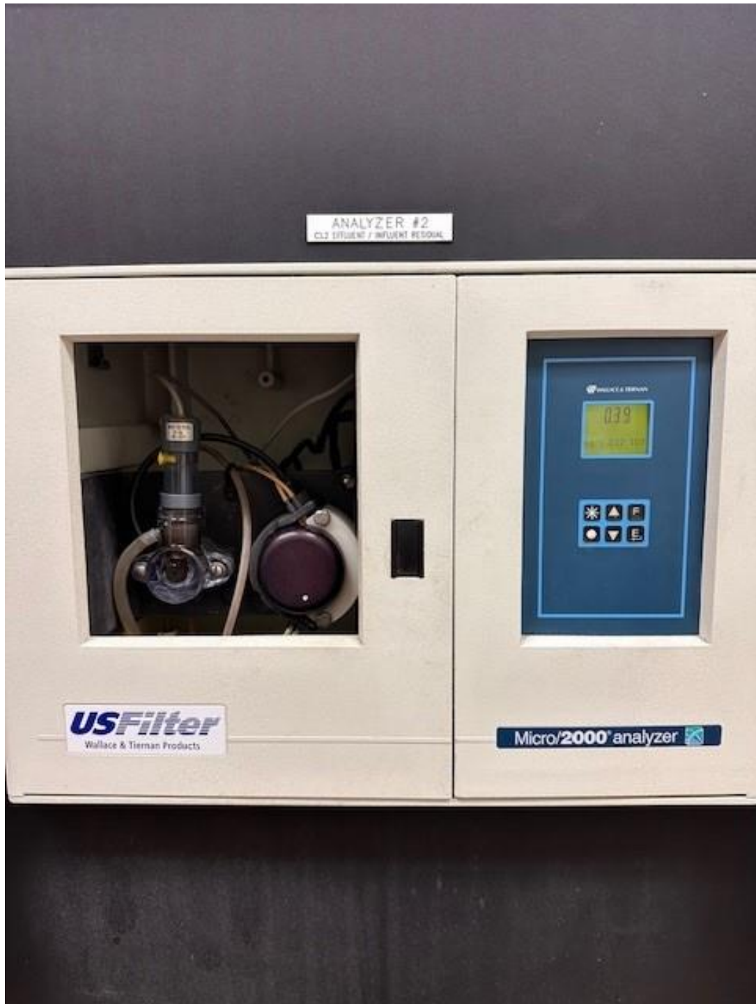
Figure 4. The effluent chlorine analyzer read 0.39 mg/L at the time of the inspection.
