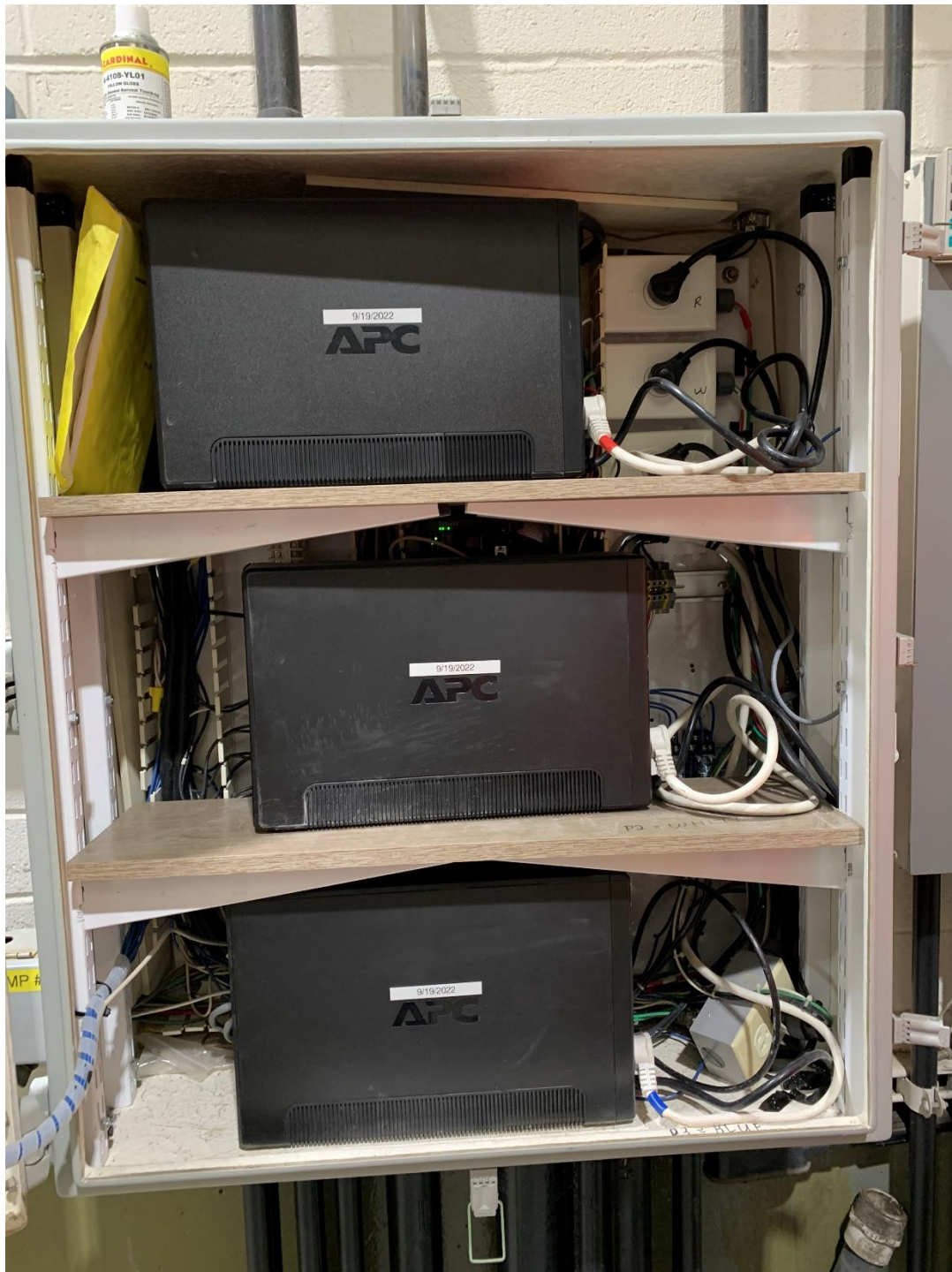
Figure 9. The three uninterruptible power supply boxes support the Facility's programmable logic controller during a power outage. EBDA last replaced these in September 2022. According to the O&M Manager, the power supply boxes are replaced every four years.
