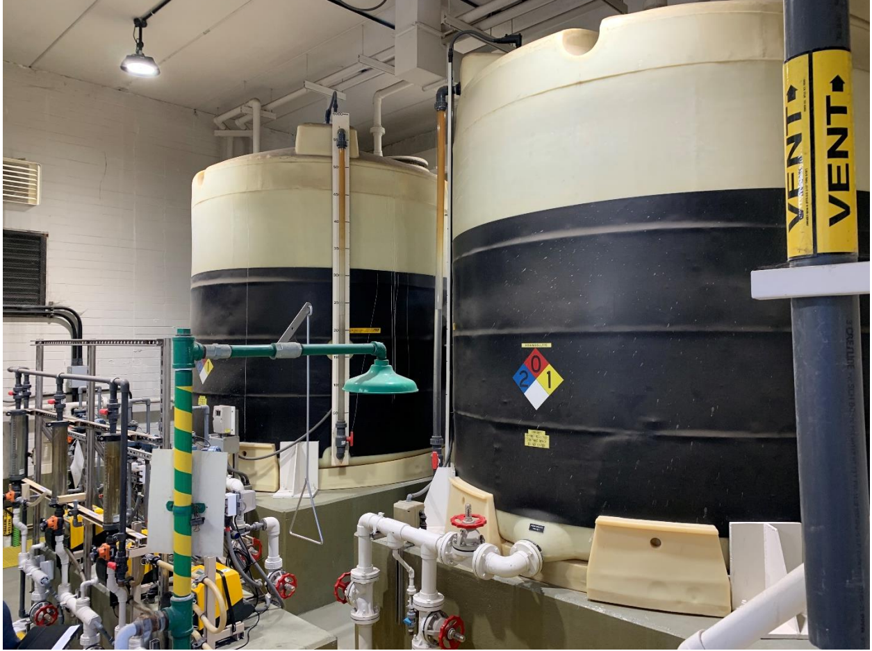
Figure 6. The Facility's sodium bisulfite storage building contained two 6,000-gallon tanks of sodium bisulfite.
