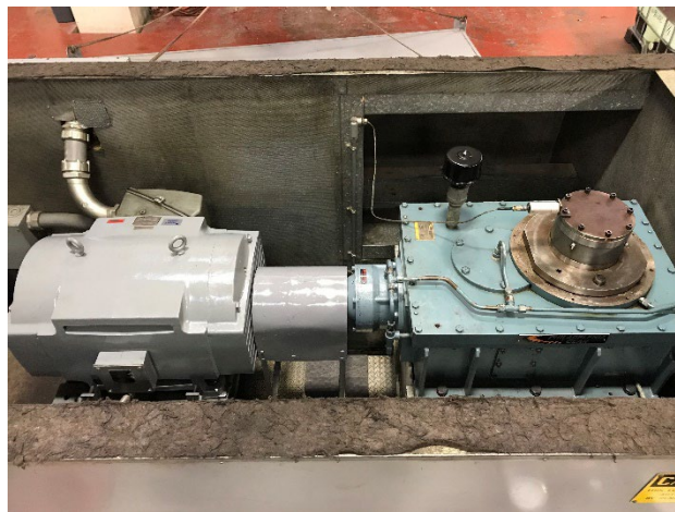
OLEPS Effluent Pump #4 Motor & Right Angle Gear Drive
