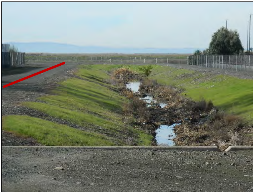
Photo 1 – View of drainage channel from Whitesell St. looking west. This channel was constructed after the EBDA pipeline, most likely resulting in locally reduced cover on the RCP force main. The EBRPD Construction Access Route will be on the south side berm of the drainage channel (photo left, red line). To photo right are the north side berm and railroad spur tracks.
