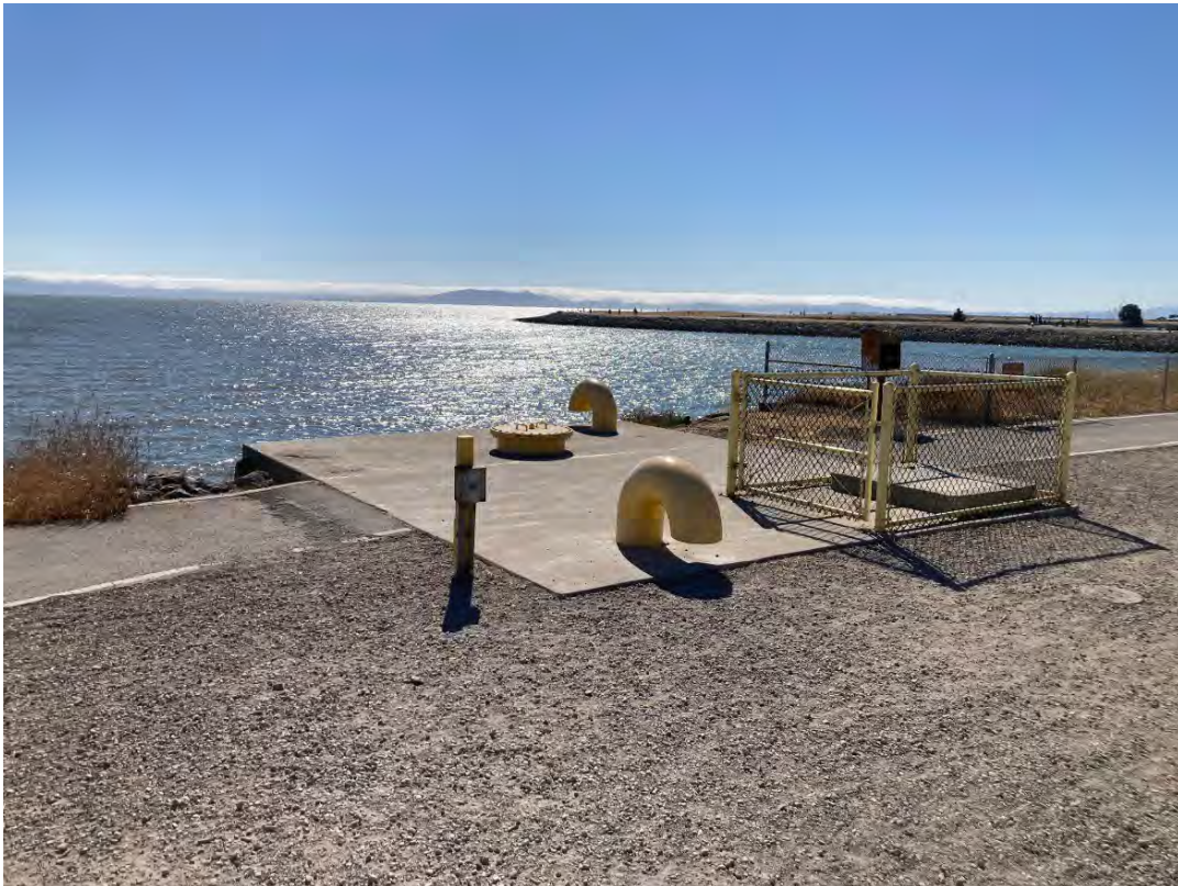
MDF Meter Vault
