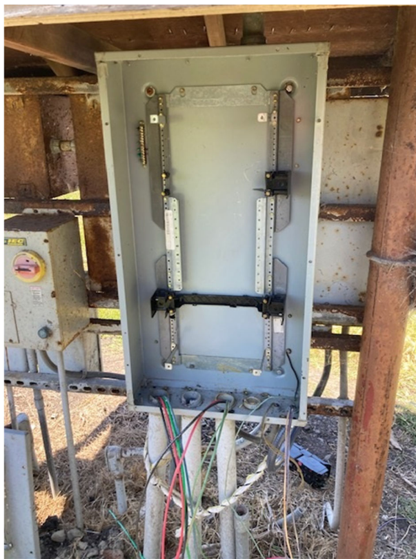
Skywest Center Pond Electrical Panel Vandalism
