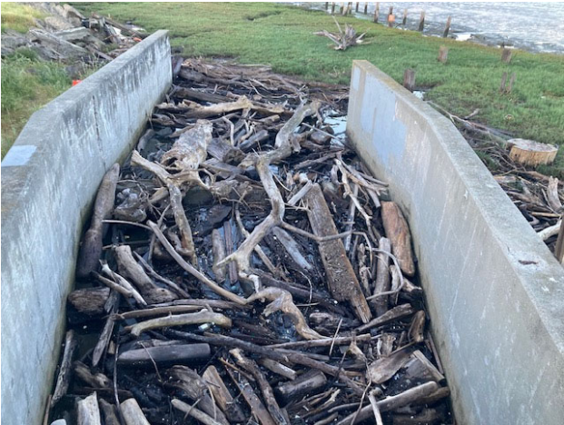
Before Debris Removal
