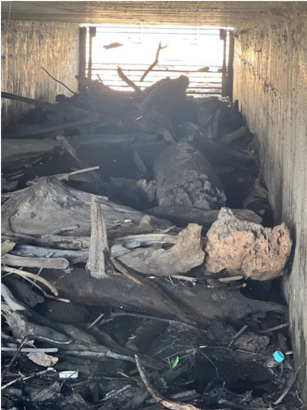
Before Debris Removal
