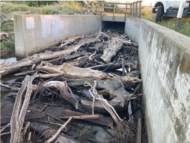
Before Debris Removal
