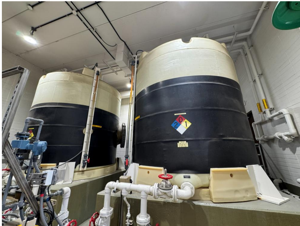
Figure 5. The Facility's sodium bisulfite storage building contained two 6,000-gallon tanks of sodium bisulfite.
