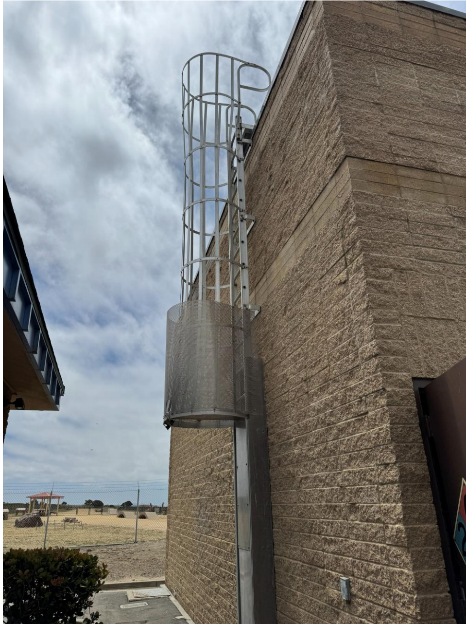
Figure 10. EBDA staff installed a guard on the ladder attached to the sodium bisulfite building.
