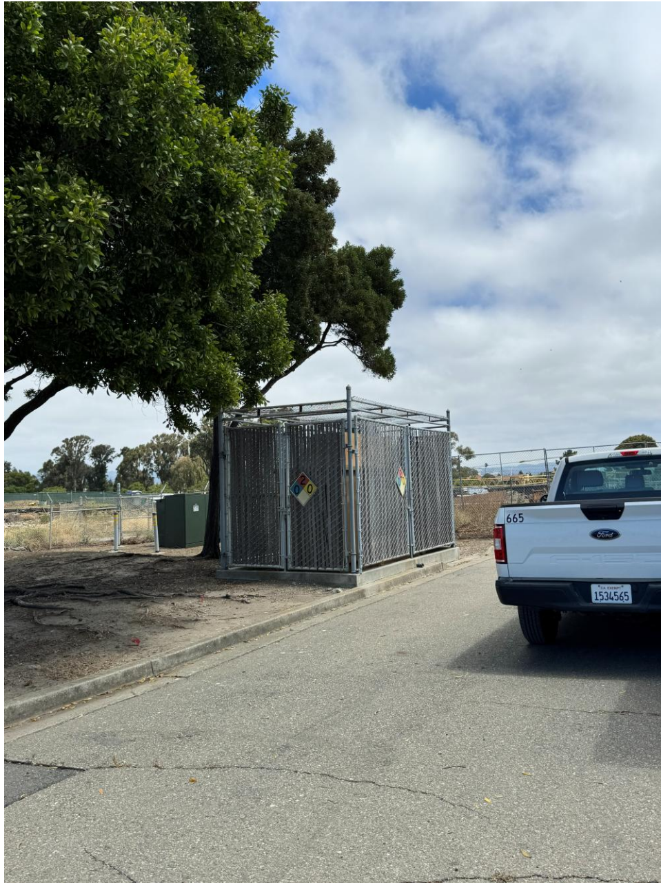
Figure 9. EBDA's backup generator was enclosed.
