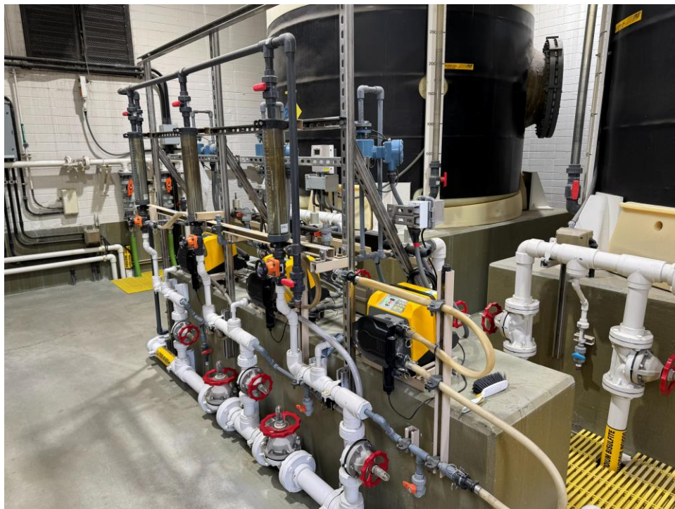
Figure 6. Three sodium bisulfite pumps.
